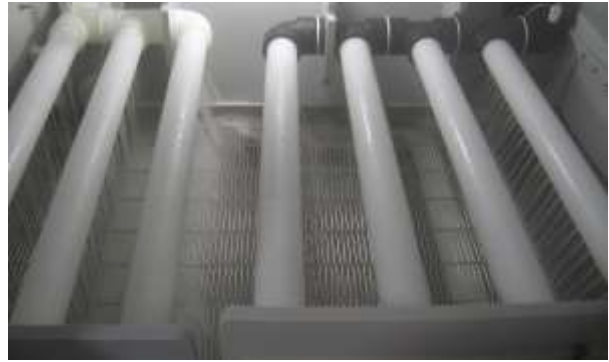
Figure 3: Picture of wash section equipped with progressive energy dynamics
